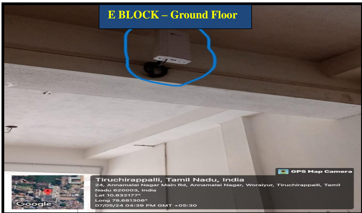
E Block Ground Floor Outdoor Device
