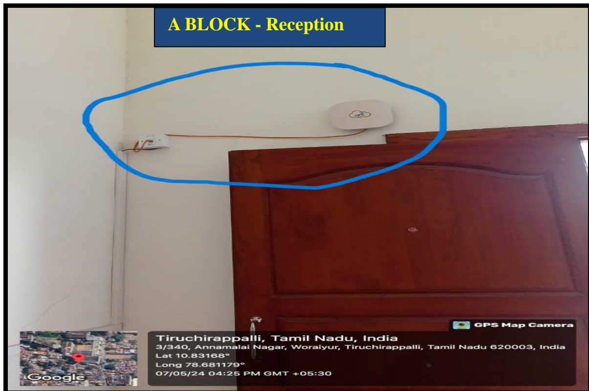
A Block Ground Floor Indoor Device
